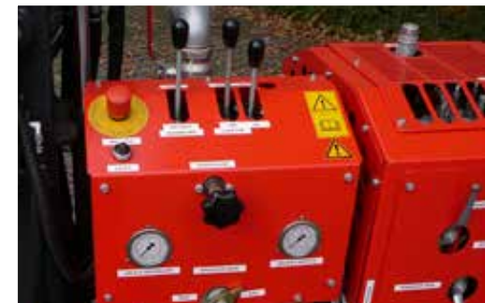
Operating station to control the drilling process
